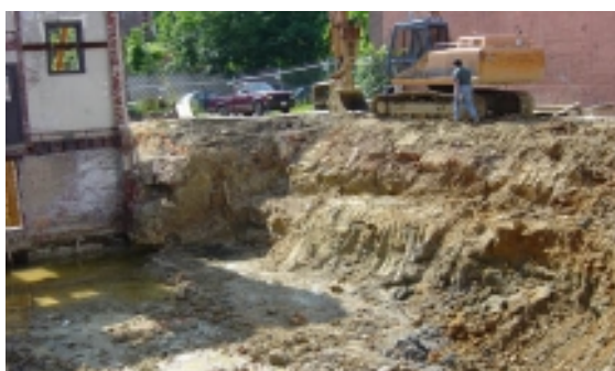
Volkert monitored the excavation of contaminated soil at Engine Company 20 prior to renovation.
