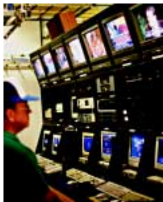
Typical MTC Control Station
